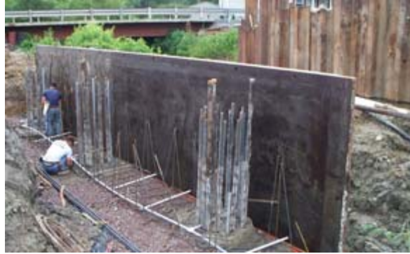
Reinforcement protruding from the tops of the three SCC caissons after completion.
