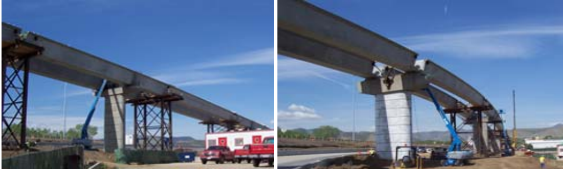
High strength, flowable concrete was used in the curved and straight girders.
